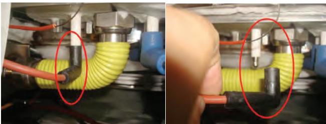
Figure 20 Flame control plug and flame control plug cable
