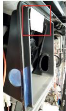
Fan is not running in the right direction
